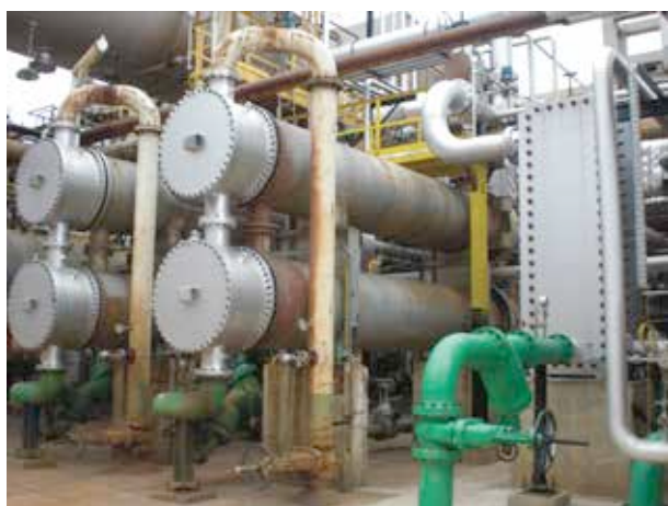
Figure 3. FCC OVHDS Compabloc installed in parallel with shell and tube exchangers.
