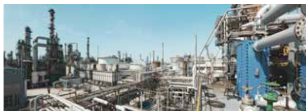
Figure 4. Crude tower OVHDS condensers preheat crude from 20 - 70 °C while condensing OVHDS to 40 °C.
